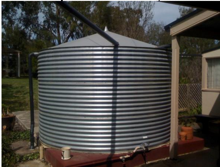
Rainwater collection water tank. Pic. Source: http://www.sustainablemelbourne.com/tag/rainwater-harvesting/
